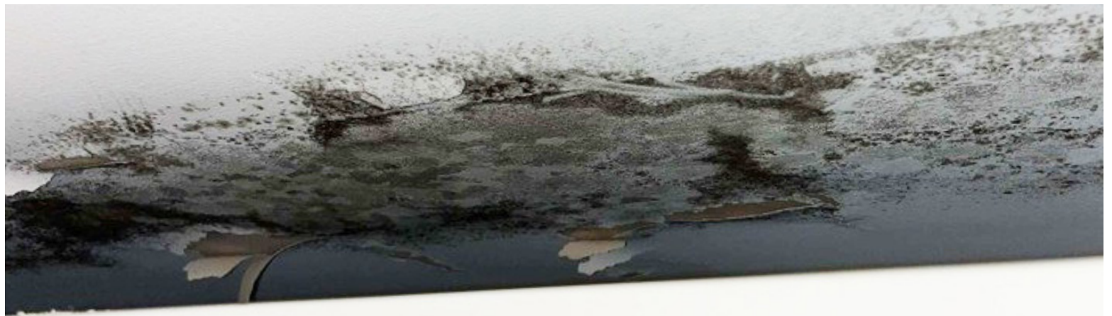
Mold in a third floor dorm room of Brannock in Elon’s Historic Neighborhood.
