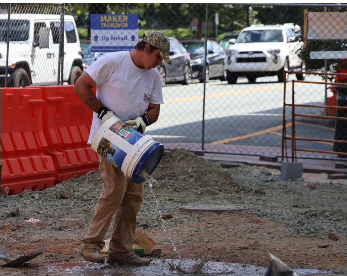
A contracted concrete worker pours water on the ground on Sept. 8 so he can make a new batch of concrete mix along North Williamson Avenue for the downtown Elon permanent plaza. According to the town of Elon, construction is set to be completed in November or December. ERIN MARTIN | VISUAL MEDIA EDITOR
